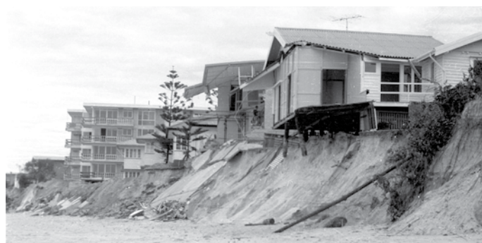
Scarping and damage to beachfront property caused by severe beach erosion on the Gold Coast, Queensland, 1967. Gold Coast Libraries Local Studies Collection.
