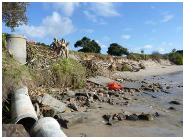
1 - Site after erosion event in 2012
