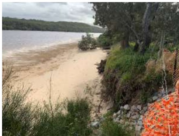
2 - erosion opposite Marine Rescue Tower threatening footpath
