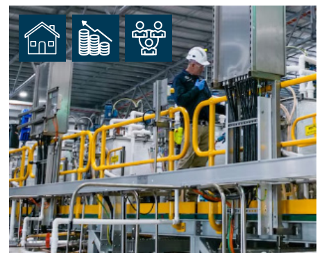
Cauldron Biomanufacturing Facility
