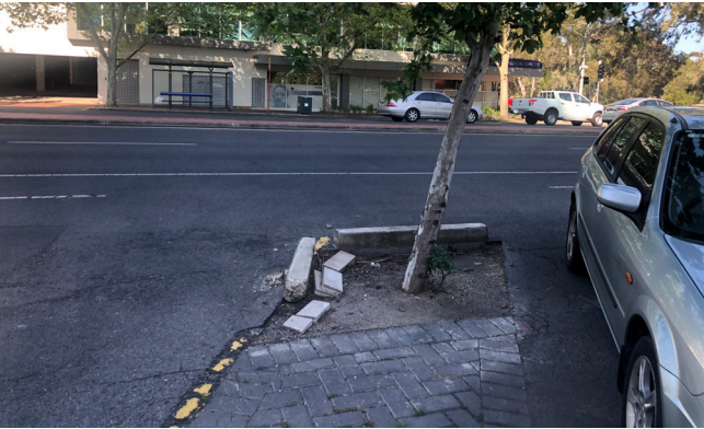
Damaged tree surrounds requiring renewal/enhancement
