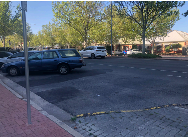
Parking bay line marking currently not to standard, resurfacing will trigger need to realign parks which may lead to minor loss of parking bays
