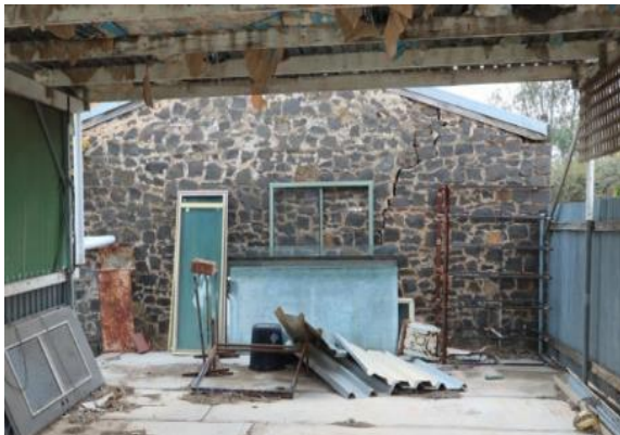
Figure 15. Bluestone rubble shed at the rear of 100 Inkerman Street as seen from the backyard of 98 Inkerman Street, Maryborough. Source: Realestate au https://www.realestate.com.au/property/98-inkerman-st-maryborough-vic-3465 .
